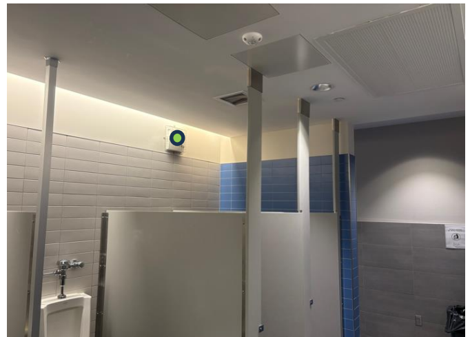
1 Sensor over 2 stalls
